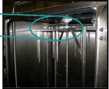
Inside Wash Chamber – Ceiling View above Rotary Deck
